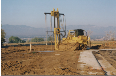
Subexcavation and moisture injection are two techniques used to reduce the effects of expansive soils.
