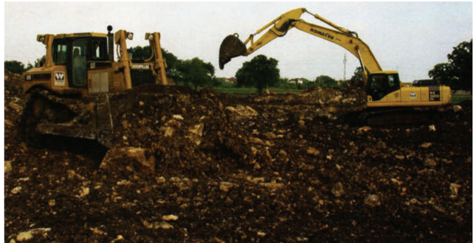
Site work recently began on the 112,000-sq.-ft. facility that will supply plastic products to the automotive industry.
