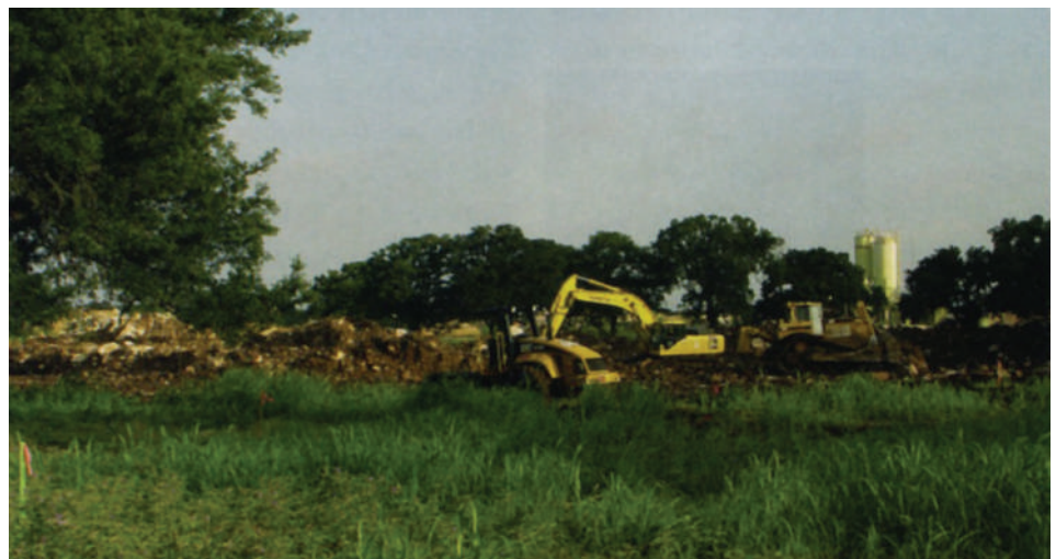
CTL/Thompson Texas LLC provided geophysical engineering for the project, which is sited on the Balcones Fault.
