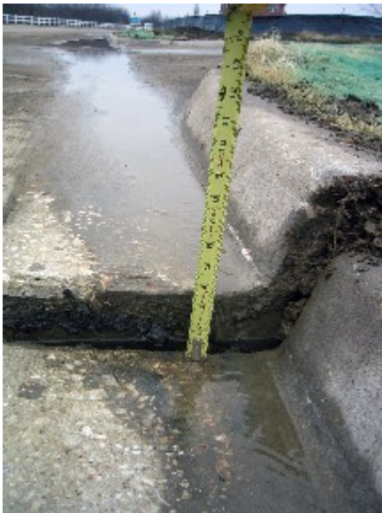
Differential vertical movement caused by expansive soil measures 3.5 inches at a pavement joint failure in the Meadow Creek subdivision in Frisco, Texas.
